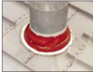
This pipe was installed in a two-piece pipe curb that allows water to drain around the pipe. By recommending a welded aluminum pipe curb, the roof manufacturer helped ensure proper installation.
