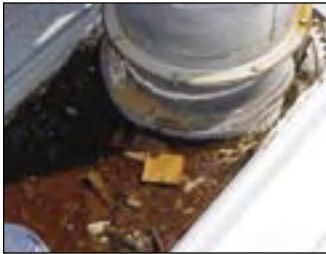
This pipe was installed in a manner that blocks the water from draining off of the roof. If the specifications do not address this, the contractor may not install it properly.
