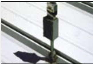
A penetration made by an electrical contractor without coordination with the roofing contractor, results in a poor penetration location which is not properly sealed.
