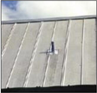
This lead hat is causing galvanic corrosion of the Galvalume® coated panel.
