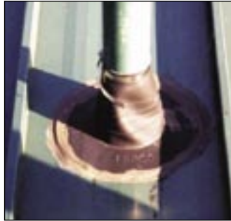
This roof jack for a rubber roof will not stay glued to the metal panel.
