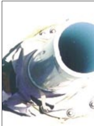
This roof jack has been ruined by sliding snow.
