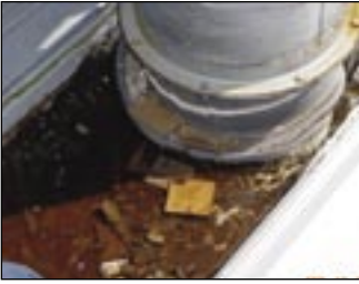
This large pipe is blocking the water from draining off of the roof.
