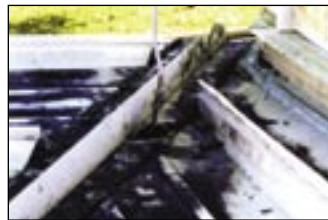
This lightning rod penetration is in the worst possible spot – in a valley where all the water is draining from the roof.
