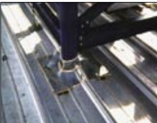
Improper flashing at structural pipe.
