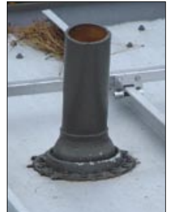
This pipe penetration has been protected from impacting sliding snow.
