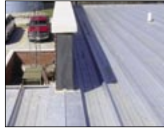
Surface caulking a flashing to a parapet wall will not provide a long-term seal.
